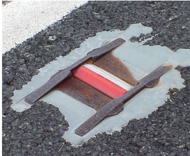
Figure 9.3 Raised, snow plowable marker system
