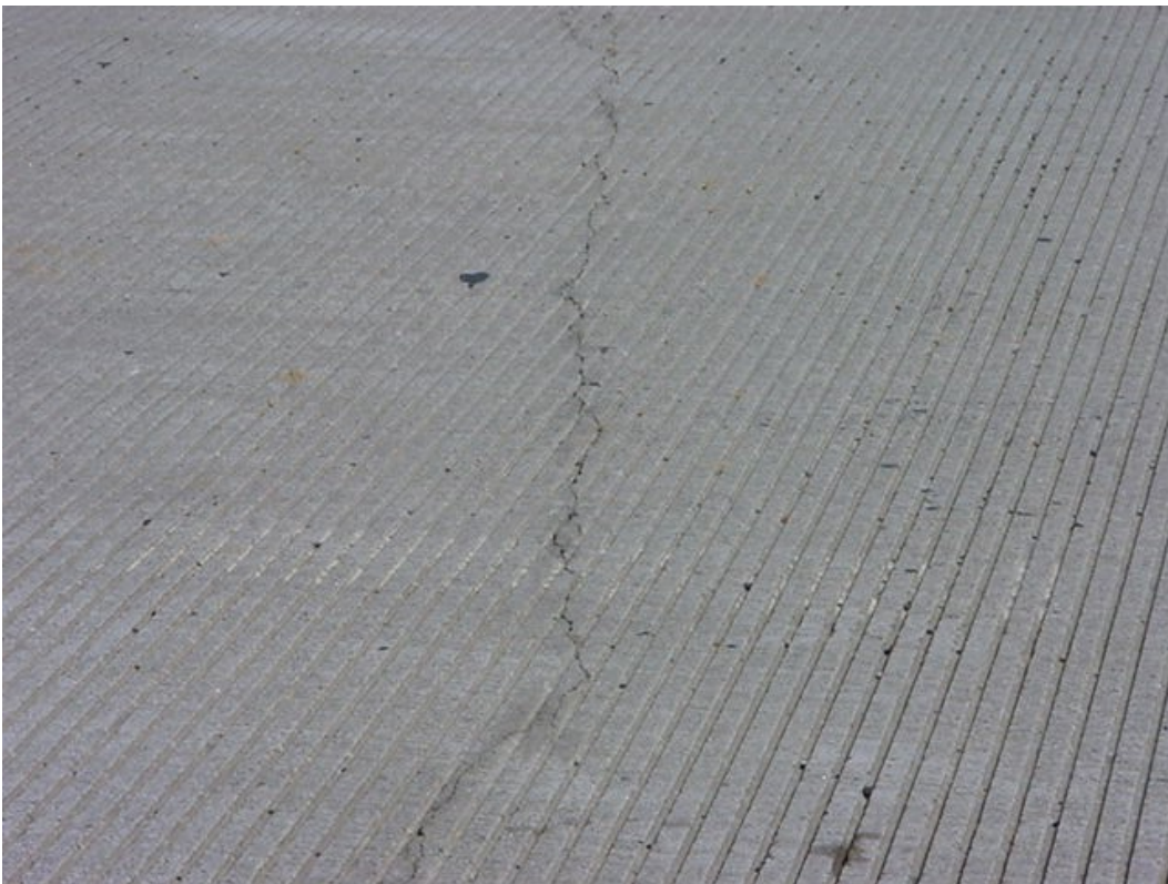
Figure 2 Deck with transverse linear cracks.
