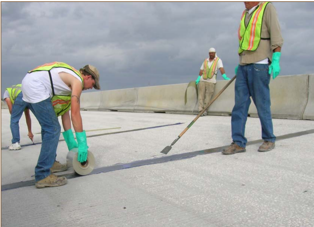
Figure 6 Carbon fiber mesh repair. Epoxy is placed on the deck surface along the crack. The carbon fiber mesh is rolled into the epoxy.
