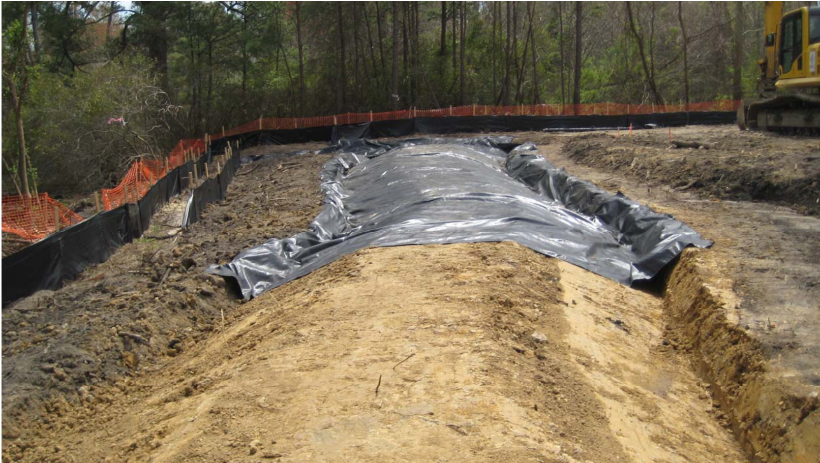
Stormwater Management Pond
