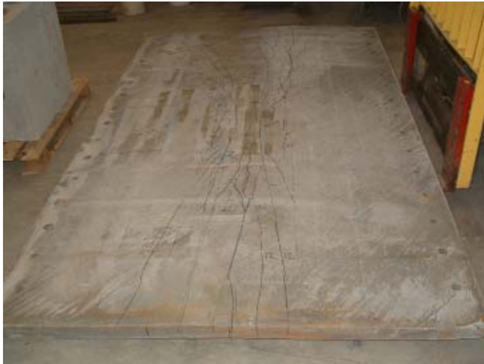
Figure 27. Typical Cracking Pattern on Bottom Surface of Large Plate Specimens.
