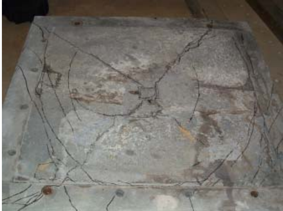
Figure 26. Cracking Pattern on Loaded Face of Specimens with Flexural Failures
