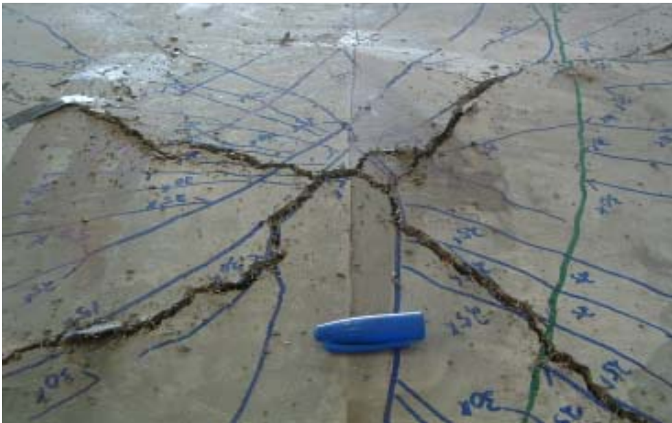
Figure 25. Crack Patterns on Tension Faces of Specimens with Flexural Failures
