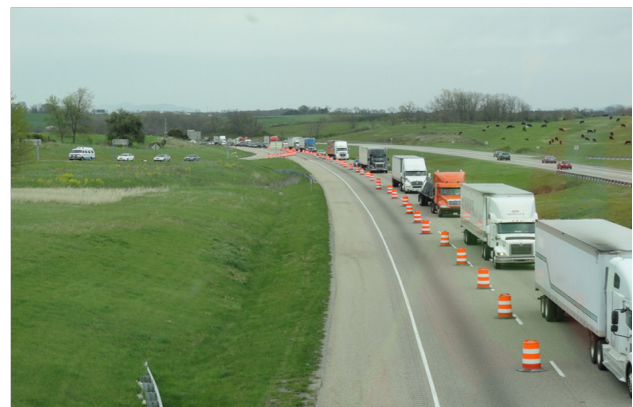
Innovative traffic management routes passenger vehicles to a primary road and channels trucks through the work zone in one lane.
