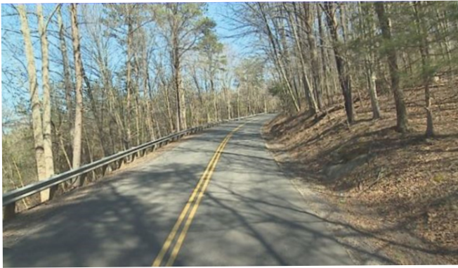
Guardrail shields an embankment slope on a low-volume Virginia rural road. (VDOT i-vision image)
