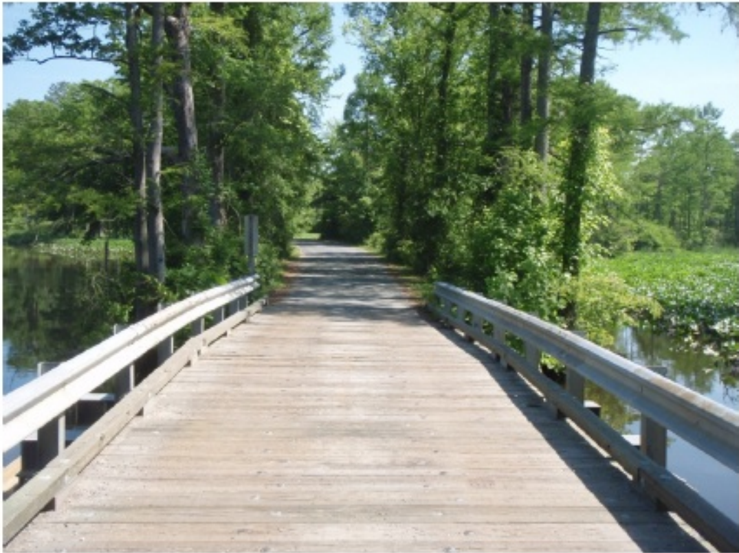
Photo Caption: This existing bridge on Route 601 (Hicks Island Road) over Diascund Creek is under construction.
