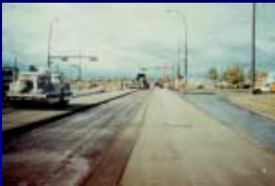
High-Volume Asphalt Intersection Milled and Replaced by RCC in 60-hour Weekend Construction
