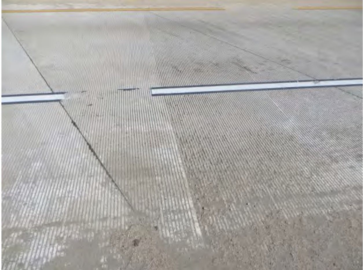
Figure 6. Scaling at Lower Portion of Photograph
