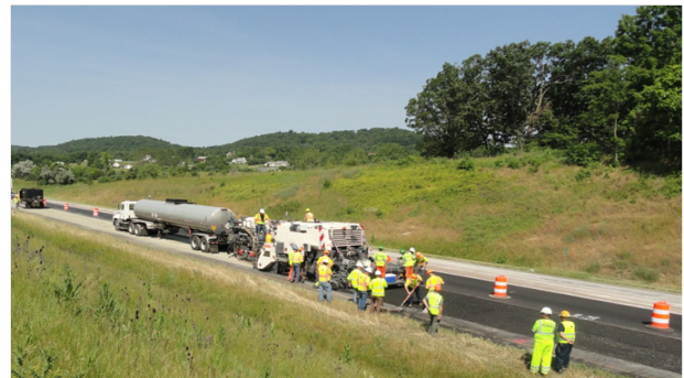
Cold in-place recycling equipment mills existing asphalt, mixes in stabilizing additives and places the recycled mixture back down in a single pass.
